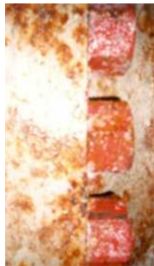
Below: Close-up of unprepared surface.
