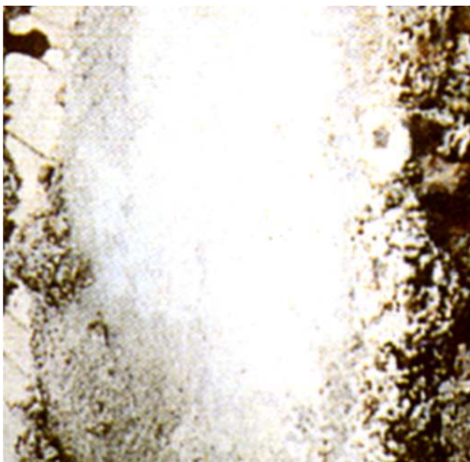
The top picture shows the heavy marine growth after submersion in the North Sea for six years. The second picture shows how the coated surface remained intact despite the hard mechanical action of the growth removal.
