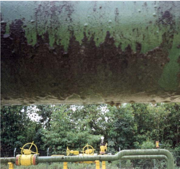
The picture above shows the algae growth which coated the surface of the pipes.
