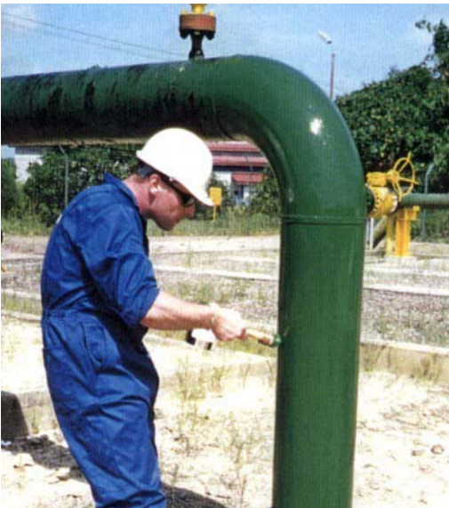
Above right, below and right: Sweating in progress during application of Alocit 28.15
