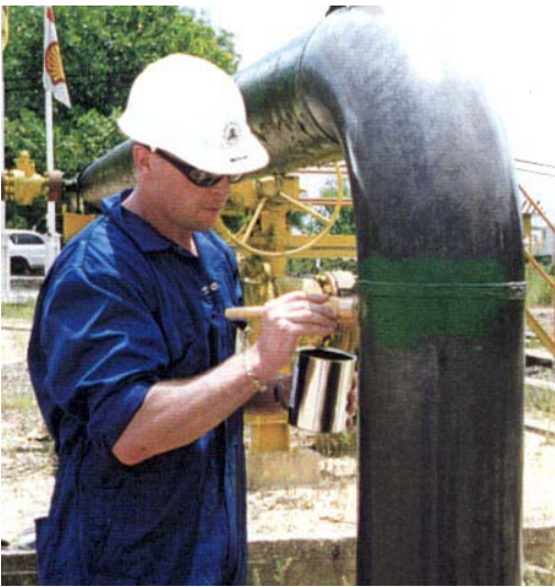
Pictured above: The application of the first coat of Alocit 28.15 Signal green
