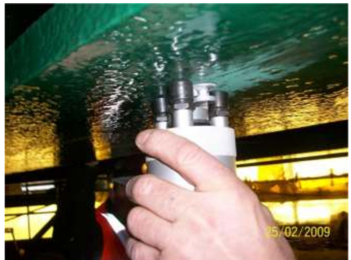
Below: Pull-off testing showed excellent adhesion with no damage to the paint surface, even at over 2000 psi!
