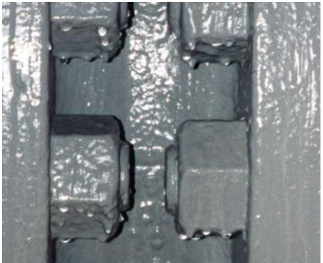
Right: This close up of a finished flange with its second coat of 28.15 Tropical Grey, shows just how much condensation was on every surface. Coating on such wet surfaces proves, beyond doubt, Alocit's outstanding surface tolerance.
