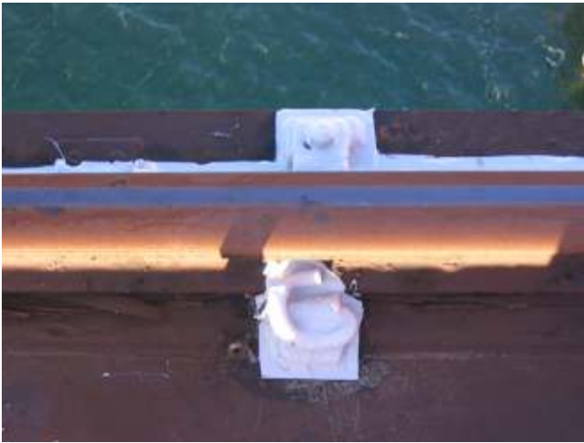
Top: A single cleat and pigtail prior to coating Above: Cleat and pigtail after being coated with Enviropeel
