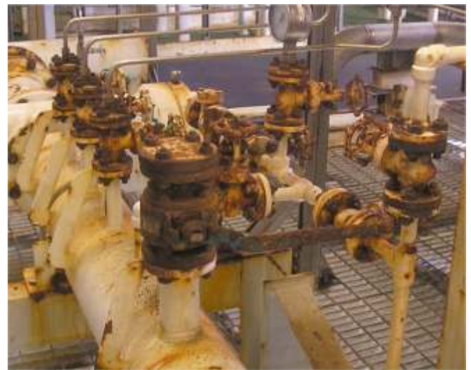
Above: a typical view of corroding flanges and valves on a North Sea platform.
